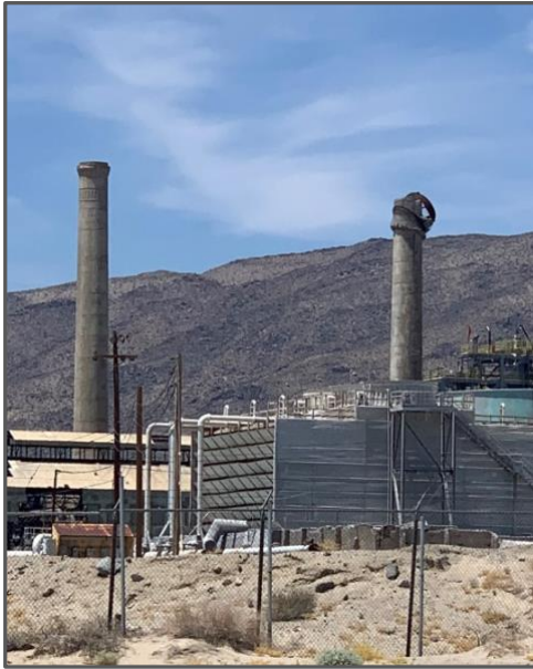
Figure 8. A displaced chimney cap at the top of the smokestack at the Searles Valley Minerals facility in Trona (right side of photo ).
