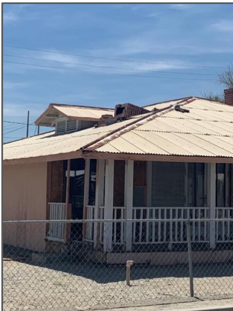
Figure 7. The chimney of this home collapsed and fell through the roof of the structure.
