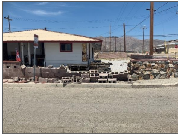
Figure 6. Damaged block wall observed in Trona. The cells within the blocks were neither filled with grout nor reinforced with rebar.
