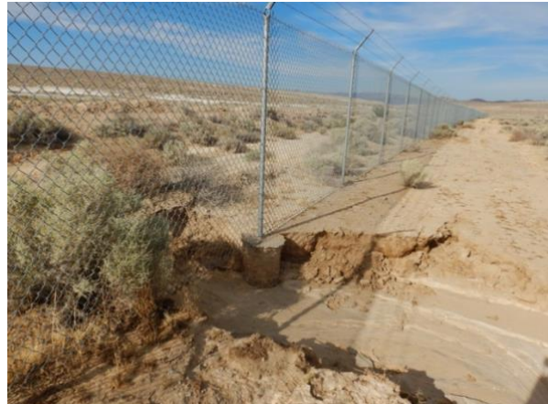
Figure 23. Evidence of scour downslope from one of the ruptured water lines along Highway 178.
