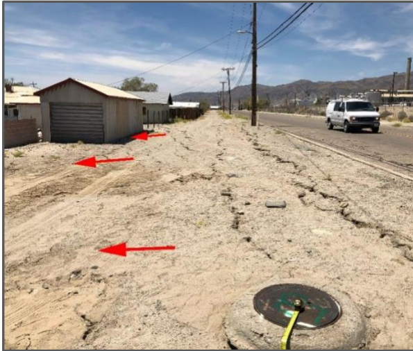
Figure 12. Lateral spreads often accompany ground liquefaction. This phenomenon occurs when drier surficial soils migrate downhill over a liquefied substrate. The spreading can take place on slopes as mild as one degree; in Trona, the affected areas slope about three degrees towards the lake (arrows showing the direction of movement).
