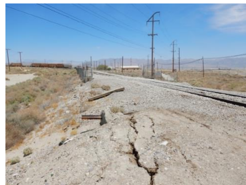
Figure 21. Private railroad line damage.
