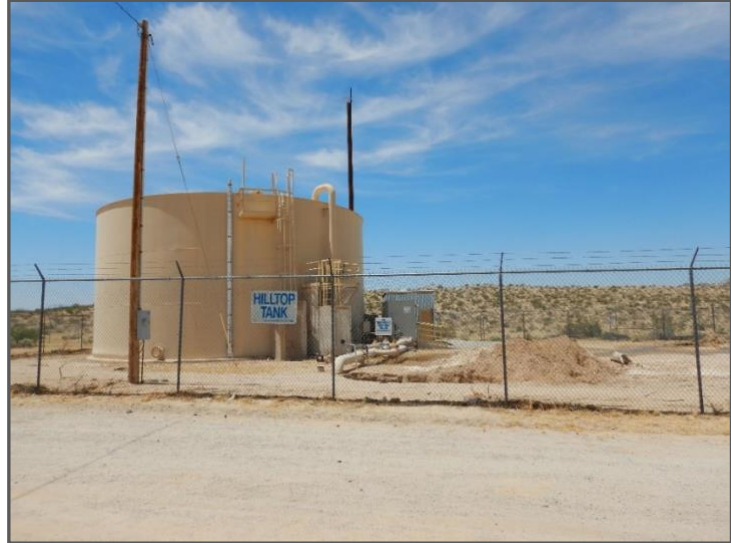
Figure 10. A pipe rupture caused water to uncontrollably flow from the tank. Evidence of the flow path is present on the right side of this photo.
