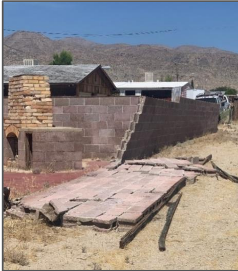
Figure 5. Damaged block wall observed in Trona. The cells within the blocks were neither filled with grout nor reinforced with rebar.
