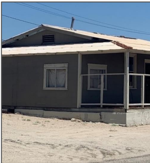
Figure 13. Lateral spreading in Trona caused damage to the foundation of this home. Ground movement occurred from left to right in this image.
