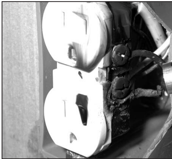
Electric receptacle failure due to a high resistance connection
